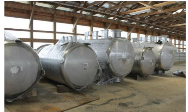
Five of fifteen nonconventional utility process tanks to be installed during conventional construction.
